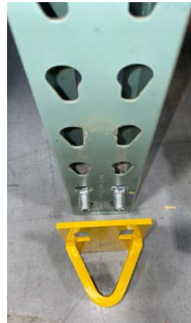
No Anchor Bolt On
